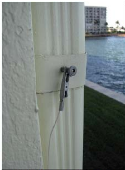
High Power Antenna Connection
